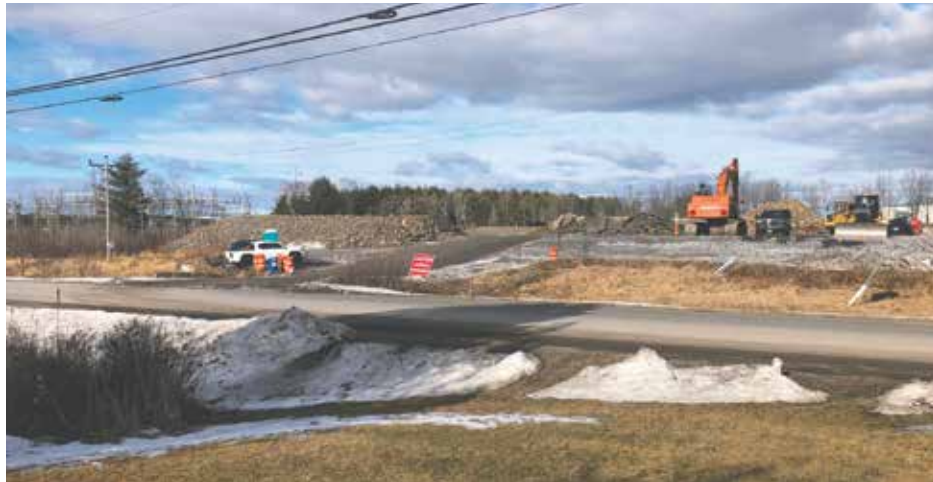
Photo credit: John Ersek Site clearing, grading, and other preparation work is underway at the five acre location where Plus Power LLC plans to build its 175 MW battery facility in the Gorham Industrial Park
